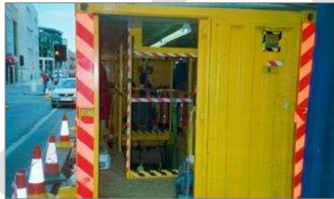
Figure 10 - HV cable jointing container
