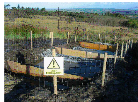
COMPLETED SETTLEMENT POND SYSTEM
